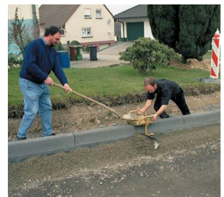
If lots of lean concrete has to be screeded an integrated hooking point for a standard shovel is provided, so a second worker can assist in pulling the device.
